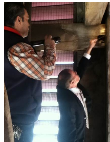
Glenn and Cesar looking at one of the beams that still needs repair
