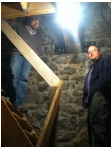
Greg and Vince looking at the new stairs going from the clock level to the next platform
